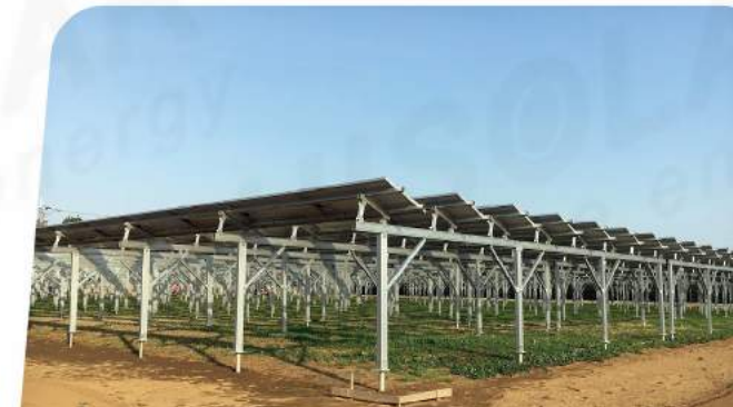
Project size: 600KW Site Location: Japan Finished Time: 2016 Project type: Solar Farm
