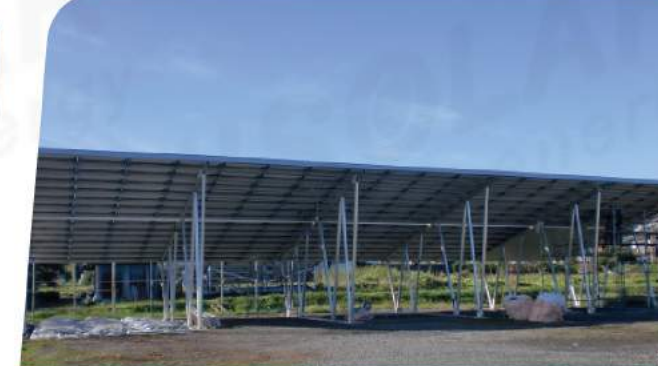
Project size: 350KW Site Location: Japan Finished Time: 2015 Project type: Aluminum Carport
