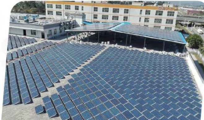
Project size: 8MW Site Location: Barbados Finished Time: 2014 Project type: Concrete Roof Mounting
