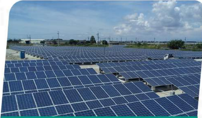
Project size: 10MW Site Location: Japan Finished Time: 2016 Project type: ST3 Aluminum Ground Mounting
