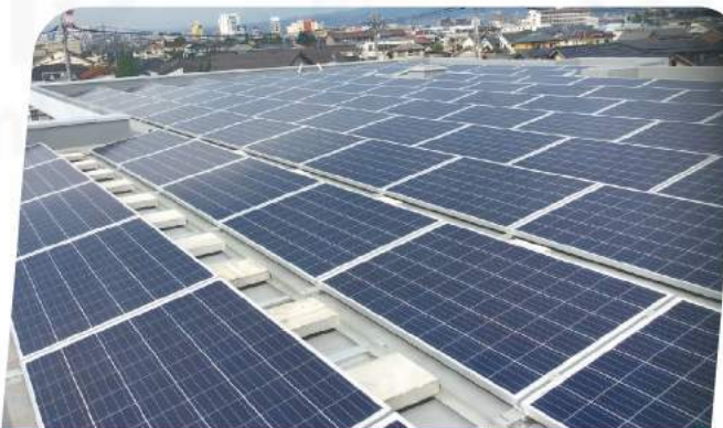
Project size: 8MW Site Location: Japan Finished Time: 2015 Project type: Ballast Mounting
