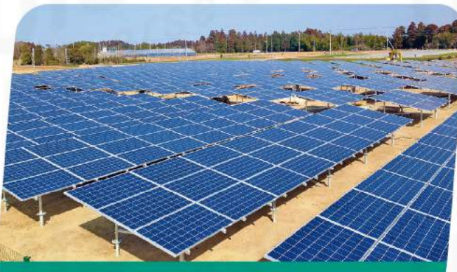
Project size: 2MW Site Location: Japan Finished Time: 2014 Project type: ST1 Steel Ground Mounting
